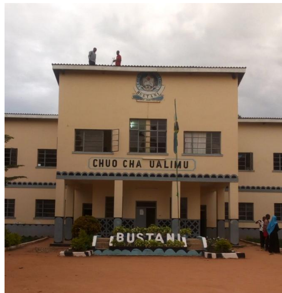
Figure 2: Installation of Customer Premise Equipment at
