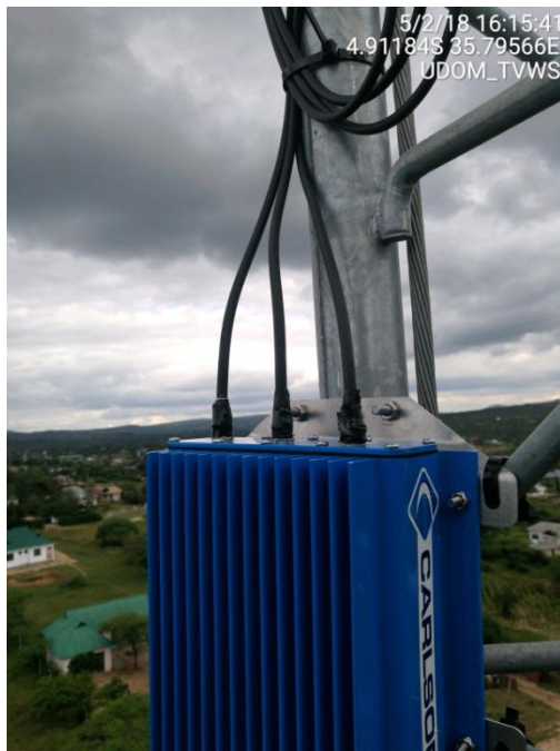
Figure 3: Base station installed at 30 Meters Above Ground Level
